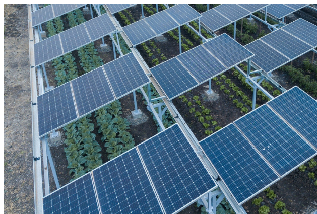
Fig. 1. An example of the agrivoltaic system on the courtyard.
